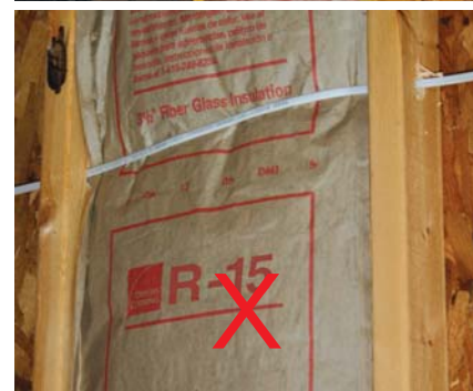
(Above) Insulation is cut/split around electrical components.
