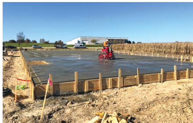
Before pouring your concrete, make sure you have all the required conduits in place. This photo of Fern Ridge Self Storage (now completed and open) show an example of a well-planned and executed site, ready for steel buildings.
