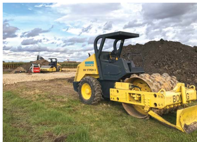
Site prep and foundation work for a two-building, 20,000 sq. ft. climate-controlled storage building expansion. Planning for stormwater handling and underground utilities for current and future phases is an important part of self-storage development.
