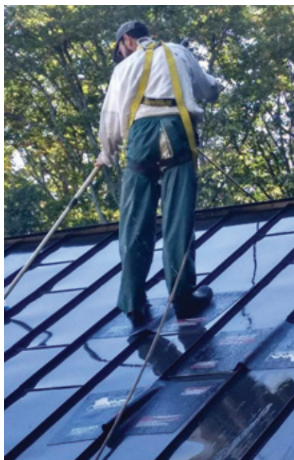
SteelGrip SAMM magnetic mats offer secure footing on metal roofs. PHOTO COURTESY OF STEELGRIP SAMM.
