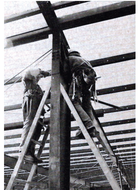
Henkel Construction Co. crewmen at work on the heavy steel beam framing stages.
