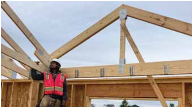
This project used trusses from Drexel Building Supply. Also visible here are MiTek connectors and Simpson Strong-Tie truss hangers.
