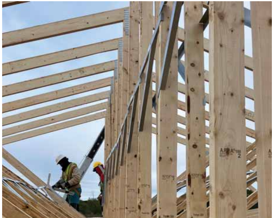
See the row of TrussBRACE pieces installed on the four webs. Unlike other braces, these don't need to be removed, they satisfy the requirement for permanent reinforcement.
