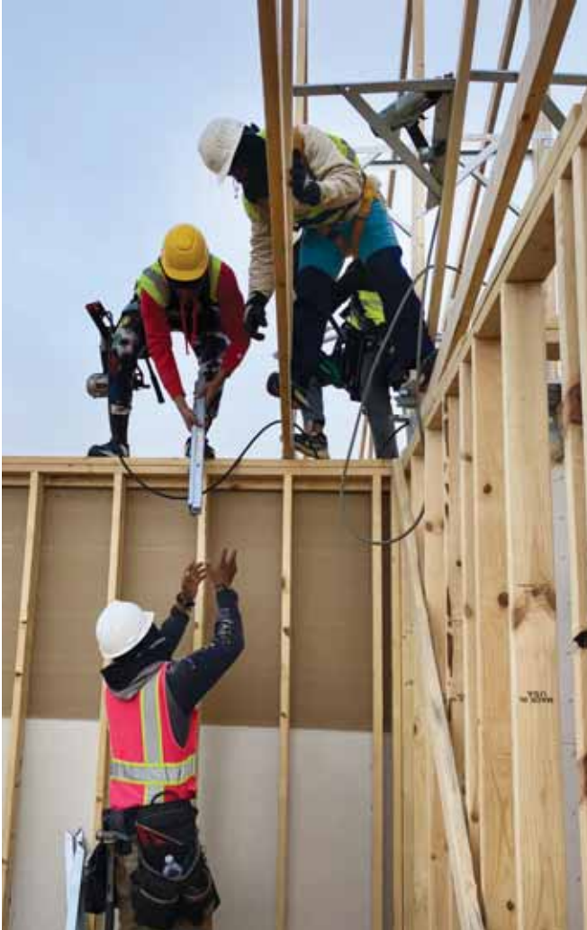
Workers will periodically hand some upward to be temporarily hung near the incoming trusses.
