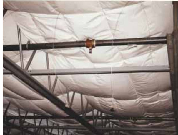
Insulation facer has sagged because the fiberglass is saturated with water. All photos by William A. Lotz
