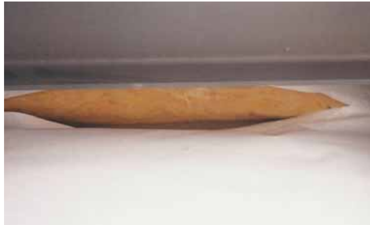
A costly mistake: This joint was never sealed.
