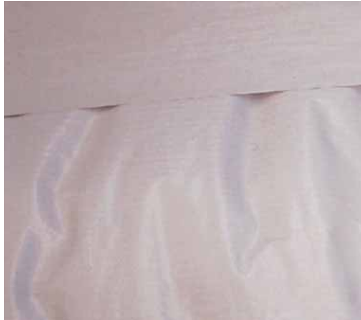
More holes in face resulting in condensation.
