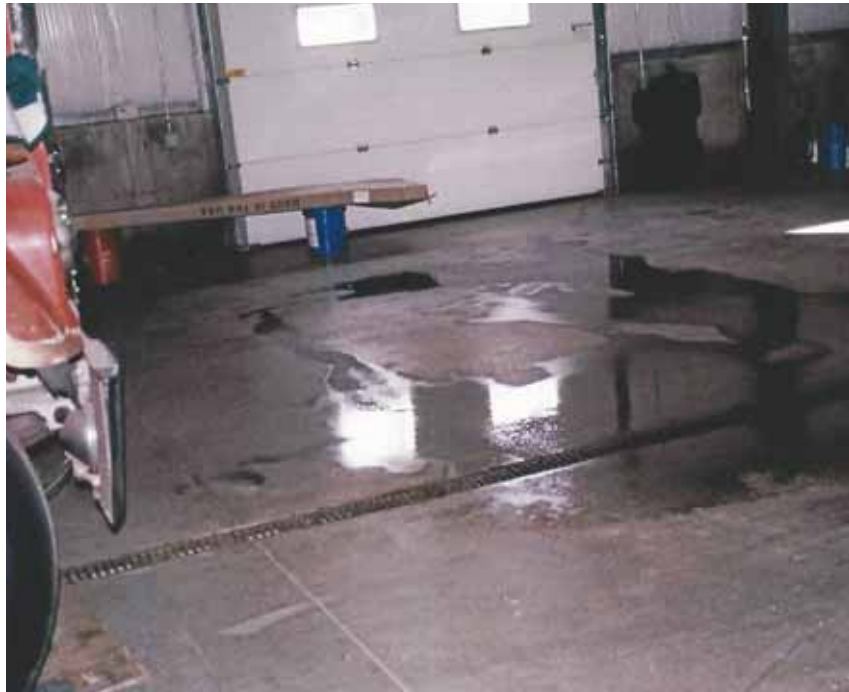
Water on the floor evaporates, the water vapor finds holes in the vapor barrier, and it rains inside the building.
