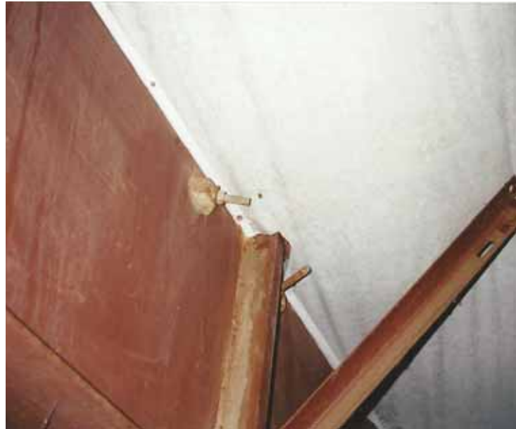
Typical holes in the vapor barrier face resulting in condensation.
