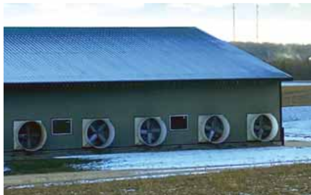
When there is a high density of livestock, adequate ventilation needs to ensure that there is no accumulation of dangerous gases, while also retaining or releasing heat and releasing water vapor.
