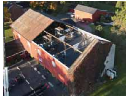
Northeast elevation during the roof demo. At this point 50% of the existing timber framing, sheathing, and standing seam panels had been removed.
