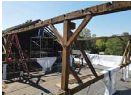
Watertight temporary flooring was installed to ensure The Barn could remain open during the restoration.
