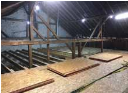
The interior of the Barn at Stratford prior to the demo of the existing timber framing.
