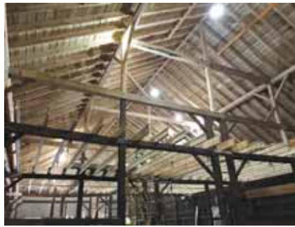
Timber framing, rafters, purlins, and sheathing were completed using post and beam construction.
