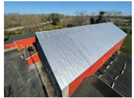
Southeast elevation upon completion of the project. In this photo you can see the pattern created by alternating sizes of standing seam panels.
