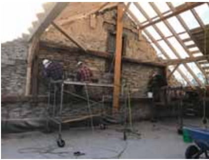
Midstate masons removed 100% of the mortar joints on the south wall and repointed them with restoration mortar to strengthen the wall and keep it watertight.
