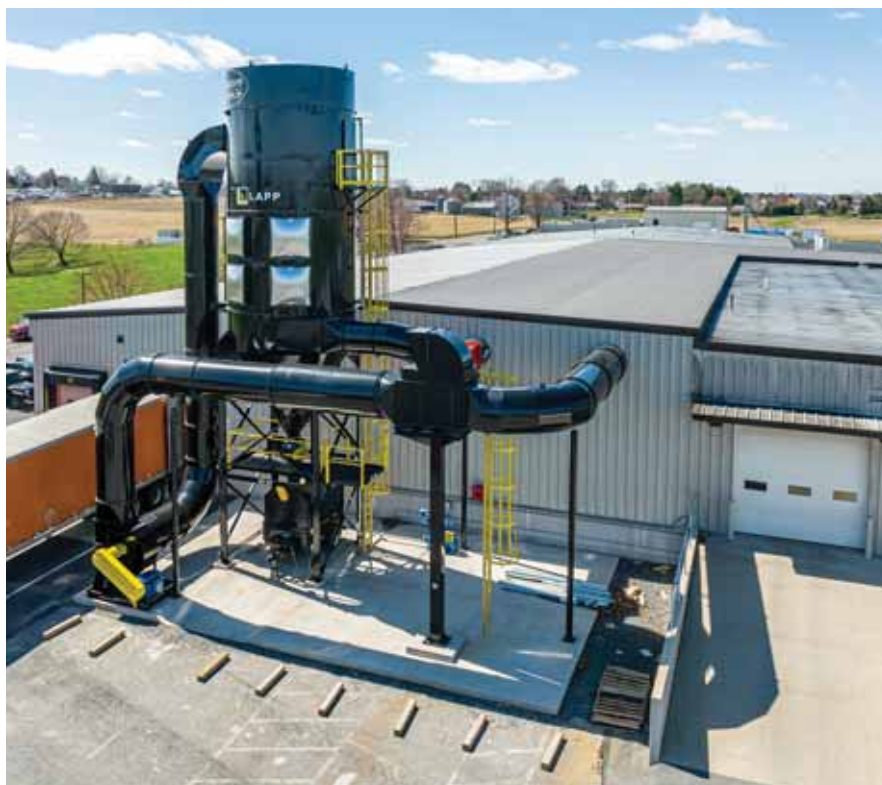
A facility dust collection system, like this one, helps ensure that working environments are clean, safe, efficient, and NFPA compliant. Each system needs to be custom designed and fabricated to meet the specific needs of the client.
