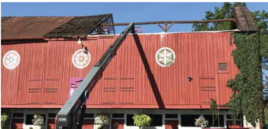
Progress of the roofing demo. This was completed one section at a time.
