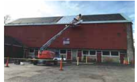
Installation of standing seam panels. Midstate began installing panels at the center of the roof to ensure the pattern is equal and consistent throughout the entire roof.
