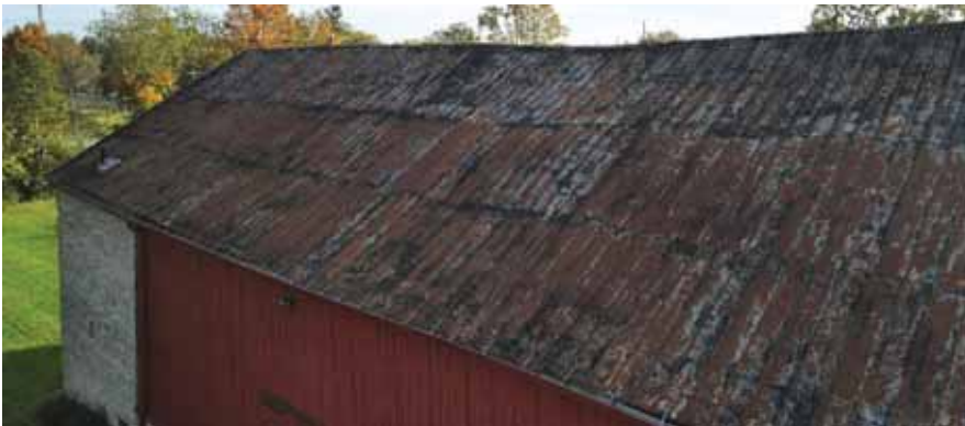
West elevation prior to Midstate beginning the demo of the existing roof.
