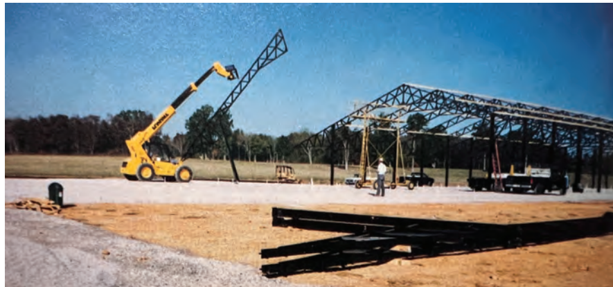
One truss assembly, bolted to its supporting column, is ready for installation and later connection to a similar opposing assembly. FRANK PAGELLO PHOTO
