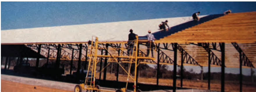
Lengths of reflective insulation are topped by full-length sheets of white steel roofing.
