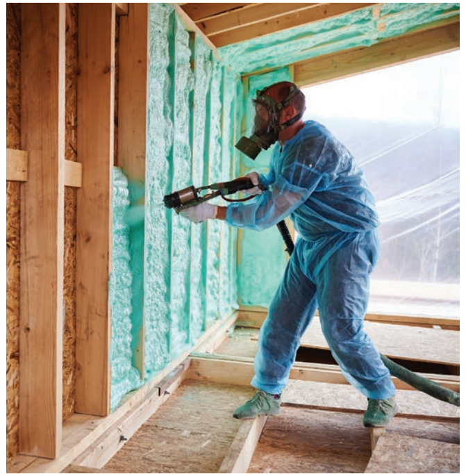
Spray foam is applied as a thick liquid that's resistant to compression after it dries to a solid. But it must be applied at a consistent predetermined thickness to meet code.
