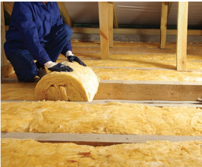
Building codes not only vary by climate zone but also for various parts of the building envelope. For example, a floor in Climate Zone 1 might require R13, while the same floor in Climate Zone 7 and 8 might require R38. AKEKSS-STOCK.ADOBE.COM
