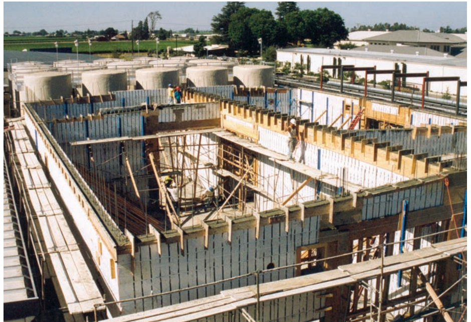
ICF walls provide a sound barrier and ambient temperature control for this 7,000-square-foot winery centrifuge and filtration building. ARXX BUILDING PRODUCTS PHOTO
