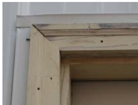
Wood jambs left unpainted, are subject to the elements and leave an unattractive, unprofessional finish.
