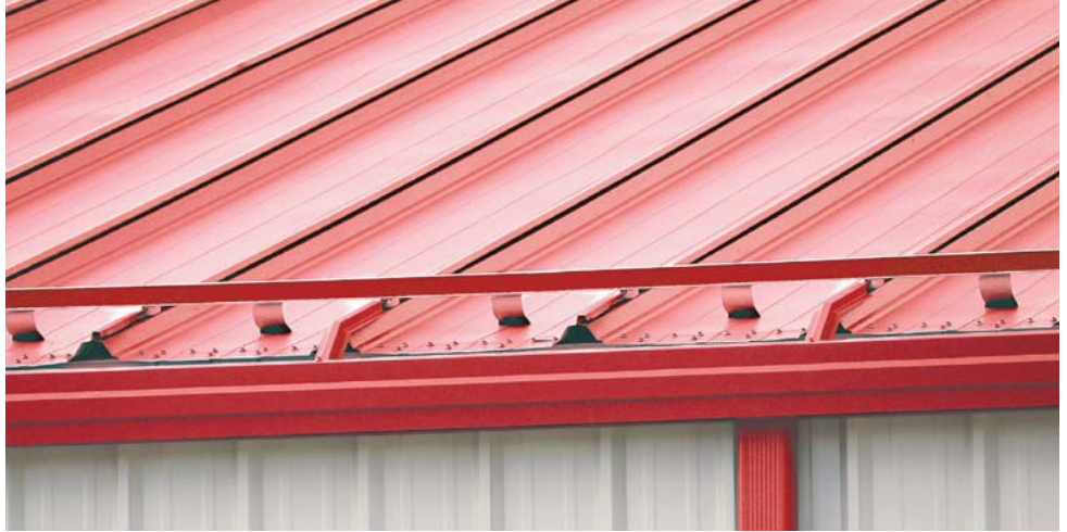
DYNA-GUARD® Snow Retention System installed on a metal roof.
