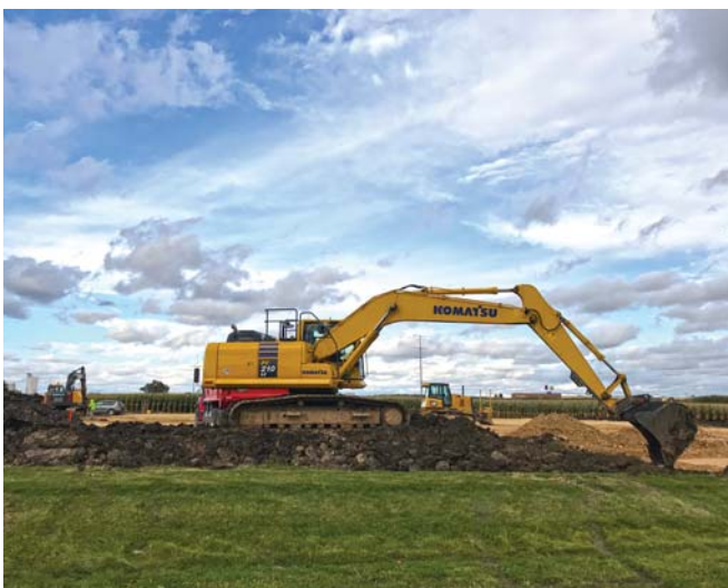
Properly preparing the build site is an important step to a successful project.
