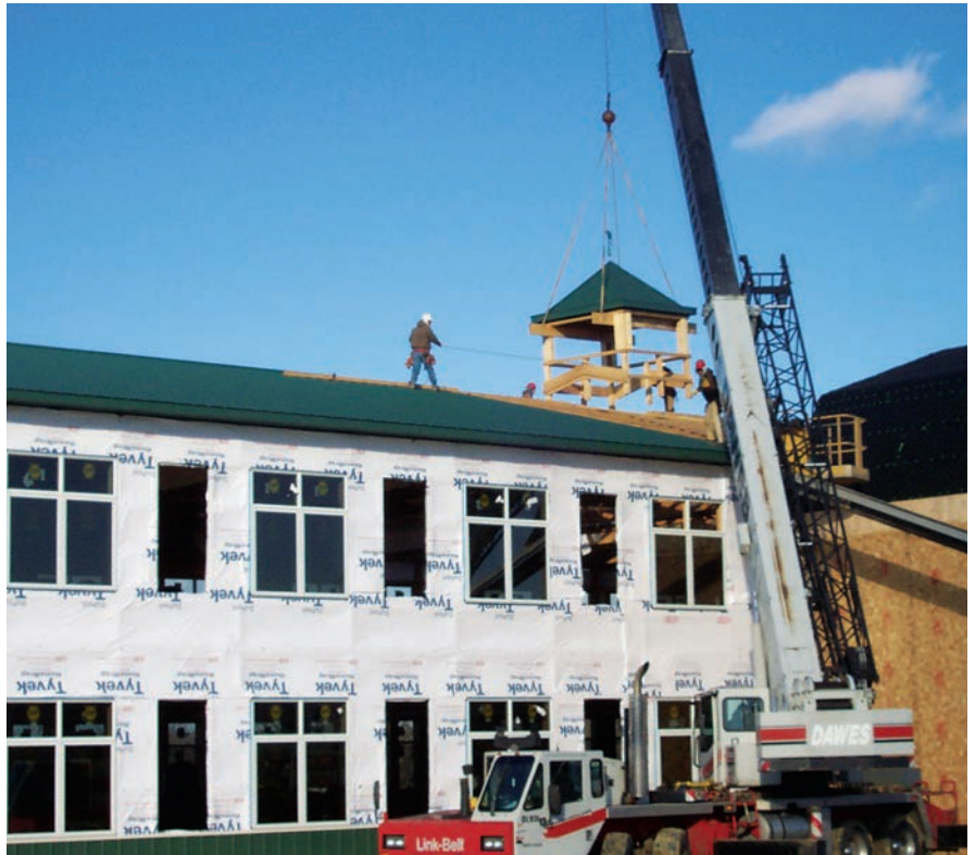
Crews guide a cupola into place atop the Organic Valley farming cooperative headquarters in La Farge, Wis. The building looks simple enough, but it is in fact as “green,” or environmentally friendly and energy conscious, a post-frame building as exists in the region. MICHAEL SCHNEIDER PHOTO
